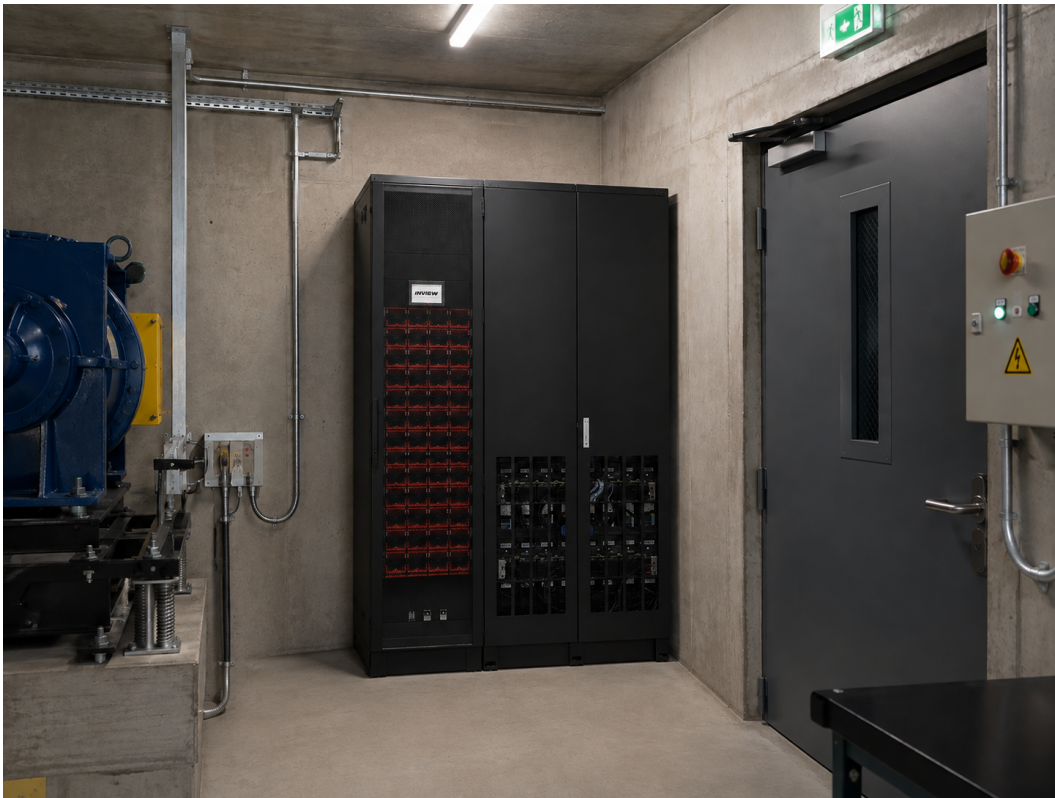
CE+T Sierra bidirectional power conversion and Inview battery cabinet installed next to elevator machinery
